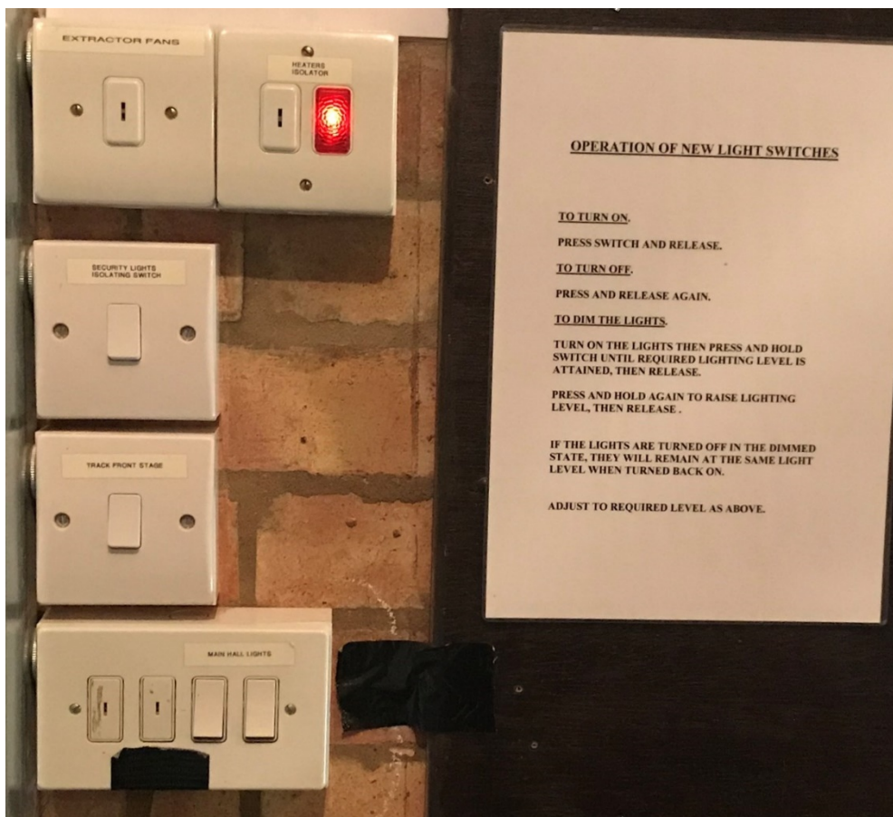
Fig 2: Lighting control panel by stage.
